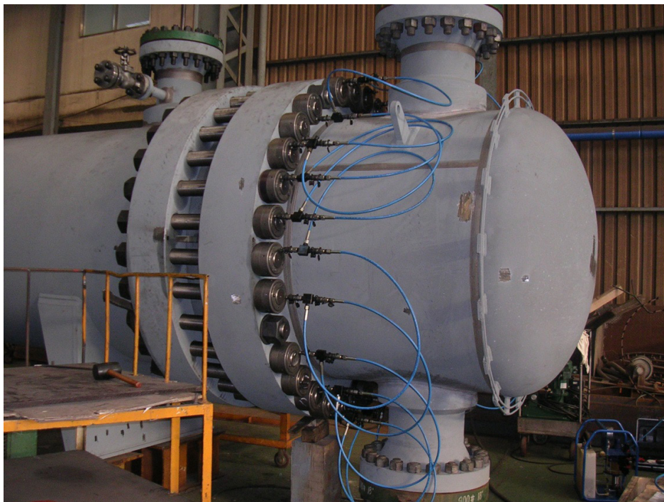
Picture Shown: Numbers of stud bolts are jacked up and tightened using jack up units at heat exchanger fabrication site.
